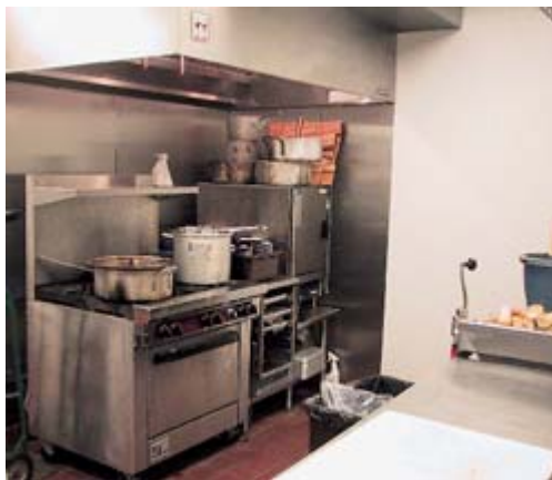
The back-of-the-house kitchen is equipped with a six-burner range, convection oven, steamer, worktables, sinks and equipment used for cook-chill production.
